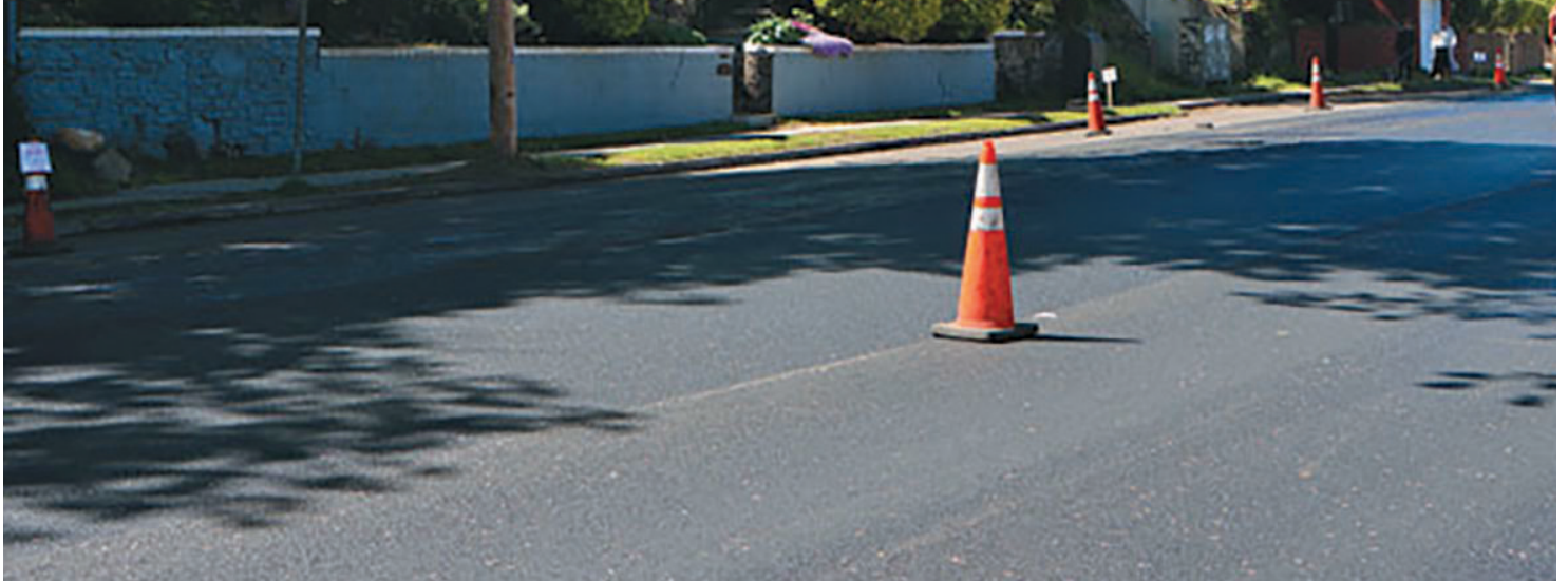
Freshly paved Kimball Avenue in Yonkers being rolled and compacted - Madison Kappel - Peckham Industries.
