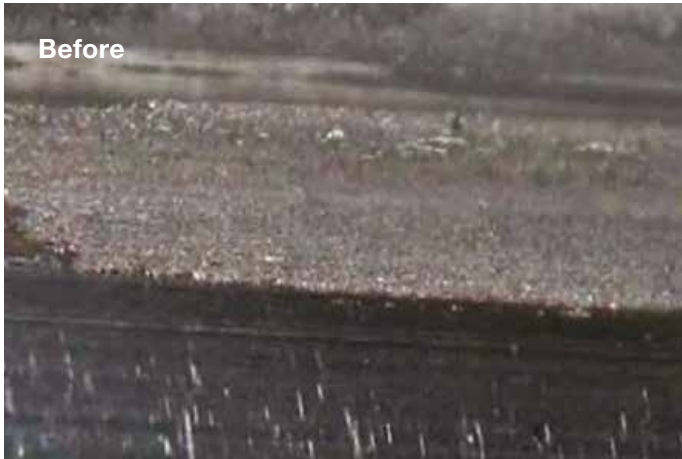
Figure 14 Micropitting and corrosion before the REWITEC application
