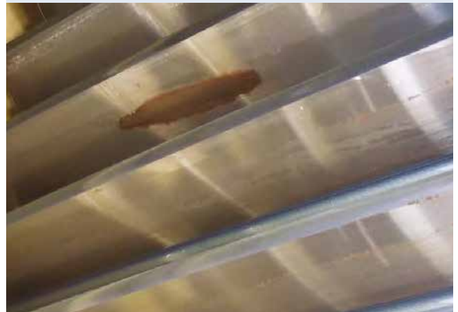
Figure 4 Visible corrosion at the tooth flank
