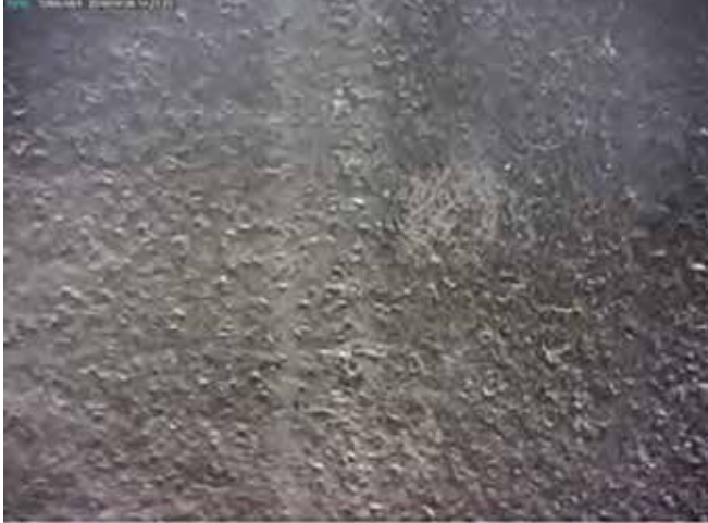
Figure 25 Before wind turbine was treated with REWITEC
